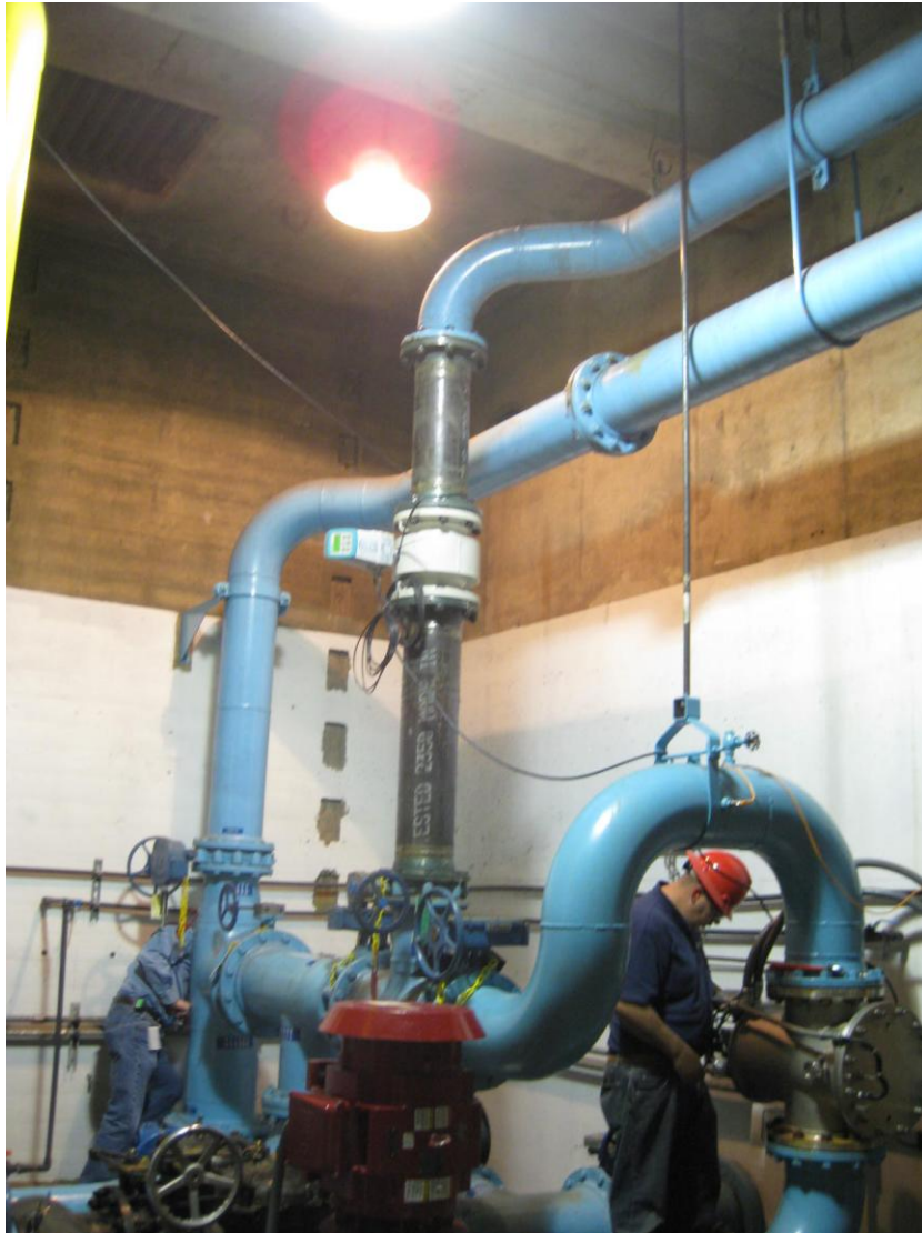
Fig.1 UV system installation in the cooling line at Hoover Dam
